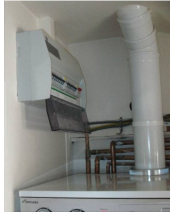
Fuse box up high
